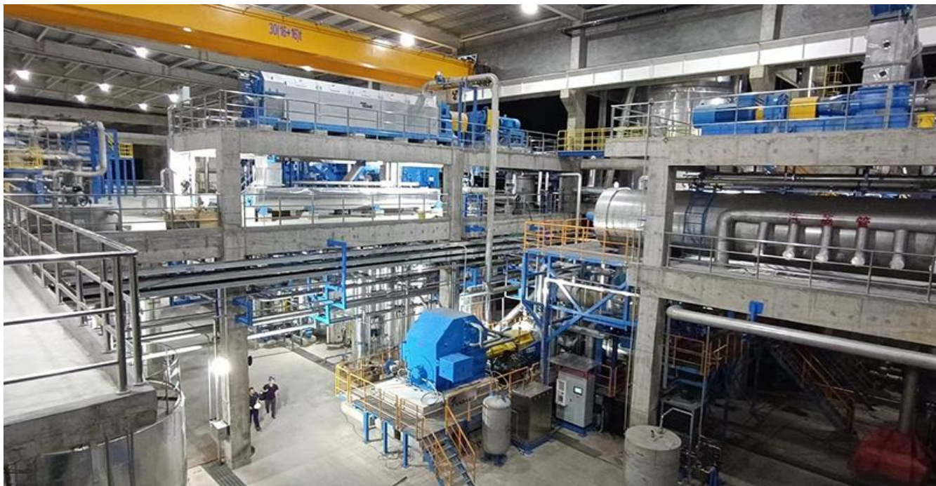
High Consistency Refiner Work Site
