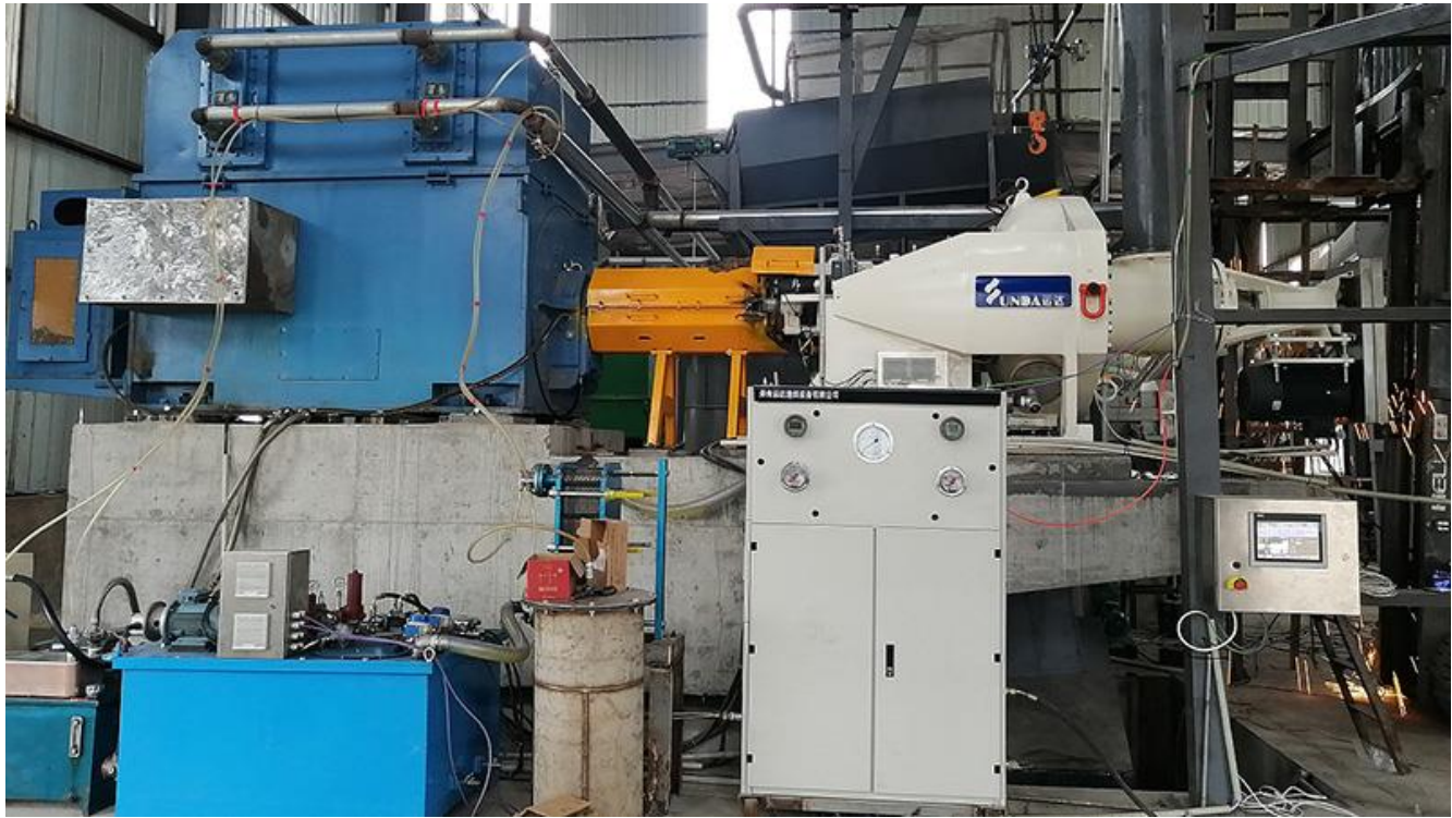
High Consistency Refiner Work Site
